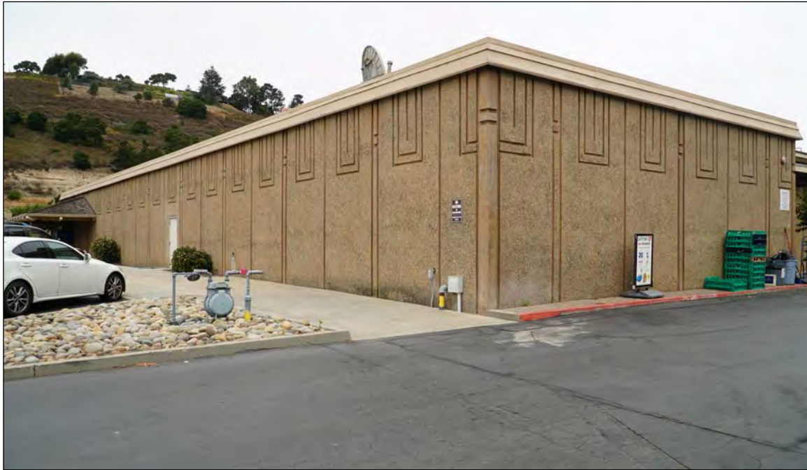
Figure 4. Looking northeast at west and south sides of Safeway, Building A, 19 August 2019.
