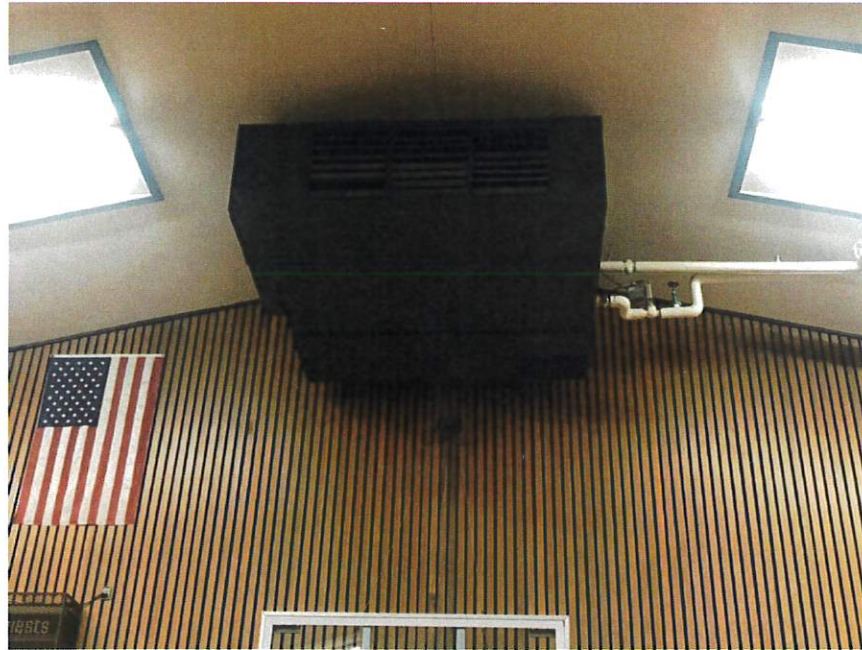
The hot air registers located inside the gymnasium at the Recreation Center.
