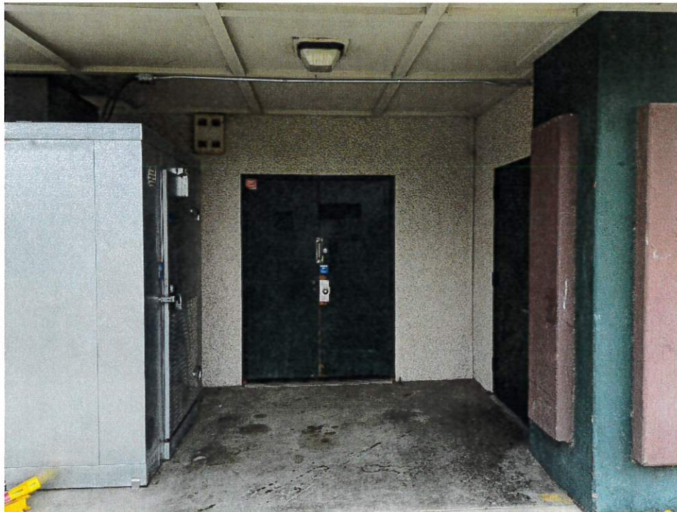
Two views of the heater and mechanical room located at the southwest corner of the Recreation Center building.
