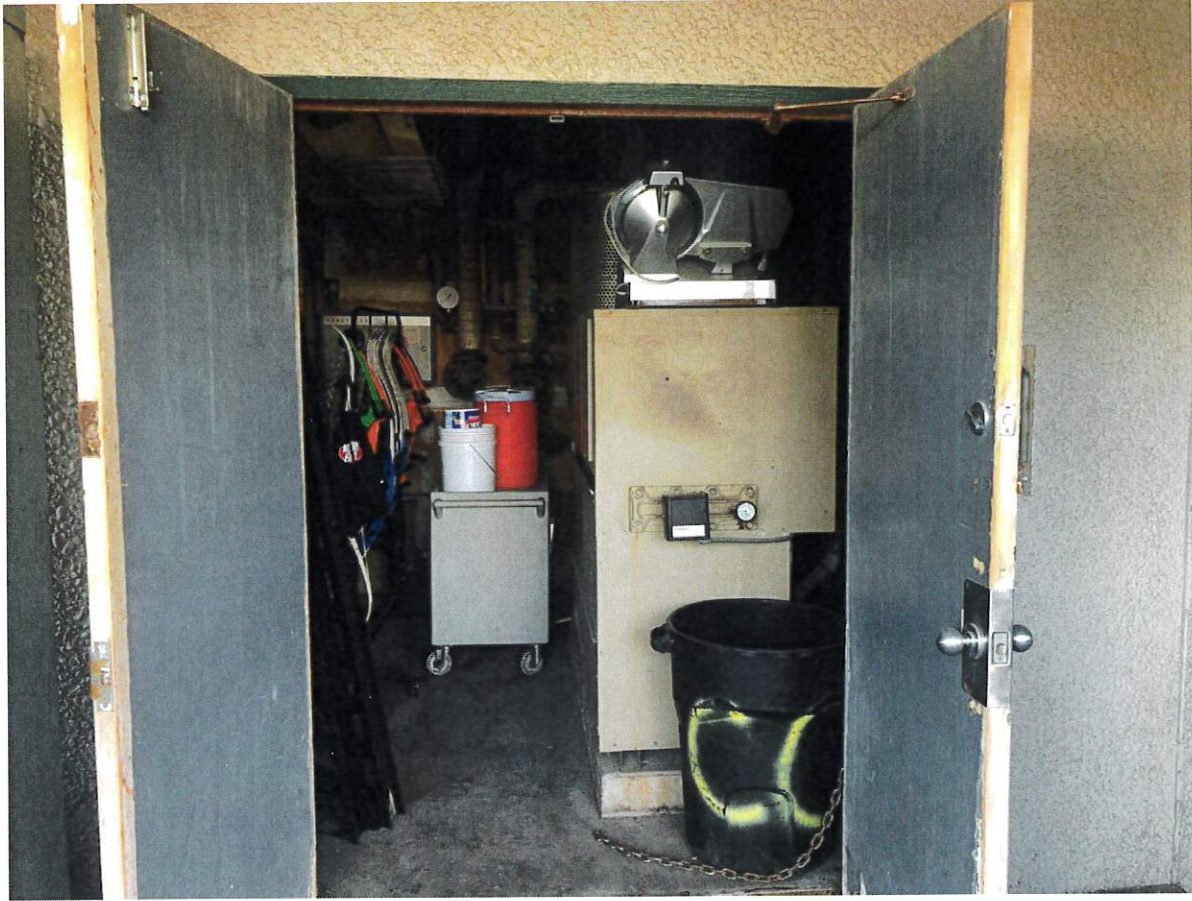
Entrance to Boiler Room from exterior of Recreation Center. The boiler is original to the building and was installed in 1968. There does not appear to be anything unique or particularly noteworthy on the sheet metal.
