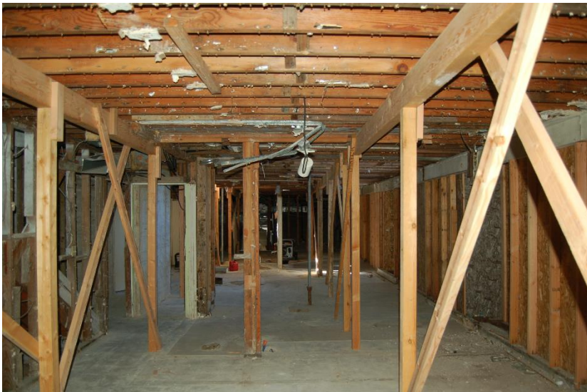
Photo 24 Lower level has been gutted of all finishes and the upper level floor is supported on two rows of wood shores.
