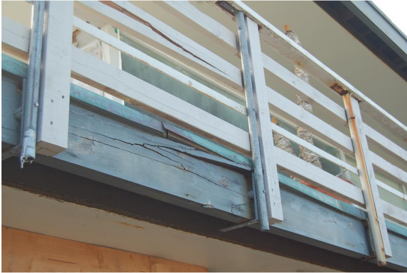
Photo 13 Deterioration and splitting at deck edge.
