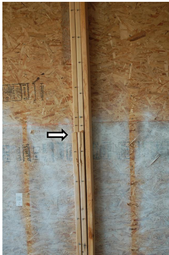
Photo 20 Failed shoring post placed at upper level north windows. New 2x member is placed adjacent to failed members.
