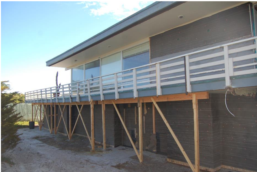
Photo 8 Exterior shoring present under west edge of deck.
