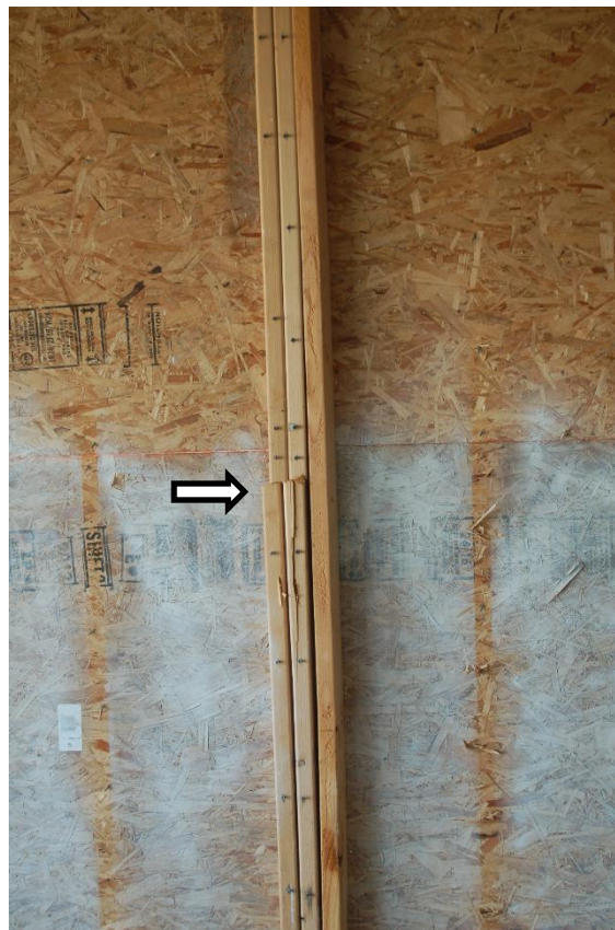
Photo 20 Failed shoring post placed at upper level north windows. New 2x member is placed adjacent to failed members.
