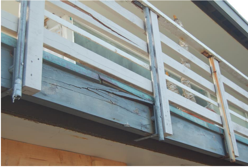
Photo 13 Deterioration and splitting at deck edge.
