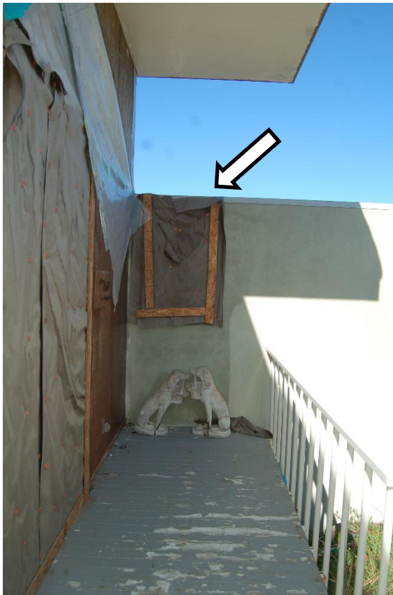
Photo 14 Damaged stucco at north buttress wall, adjacent to house.
