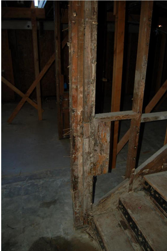
Photo 23 Water staining and damage to wood framing at lower stair.
