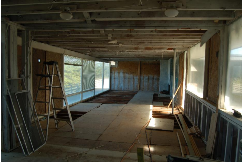
Photo 15 The interior of the upper level has been gutted with much of the flooring removed.
