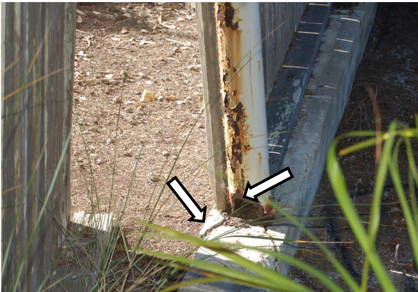
Photo 28 Hole at base of cantilever pipe fence support and spalling of concrete curb.
