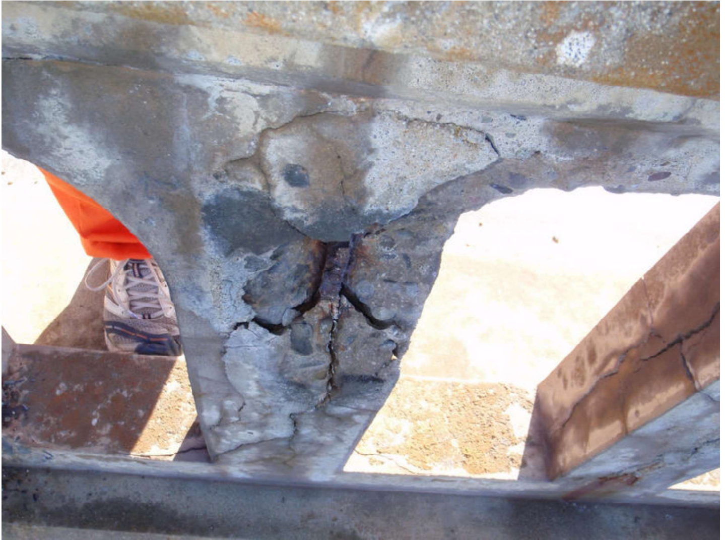
Photo #7 Gross deterioration of bridge railing.
