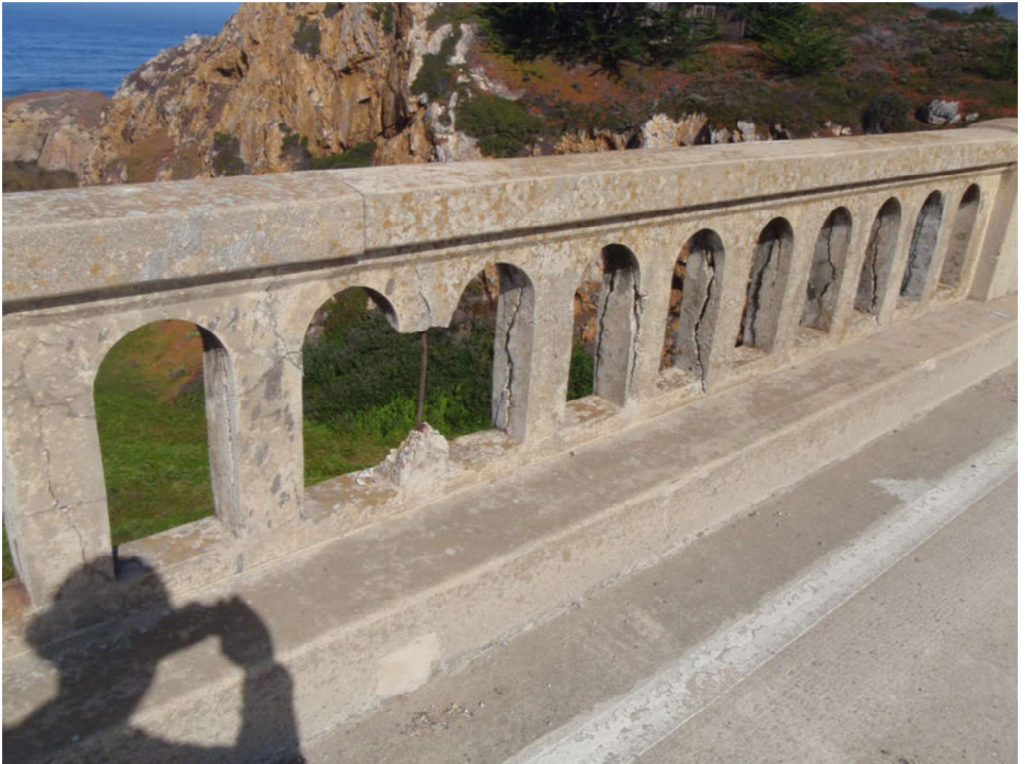
Photo #4 Gross deterioration of bridge railing.
