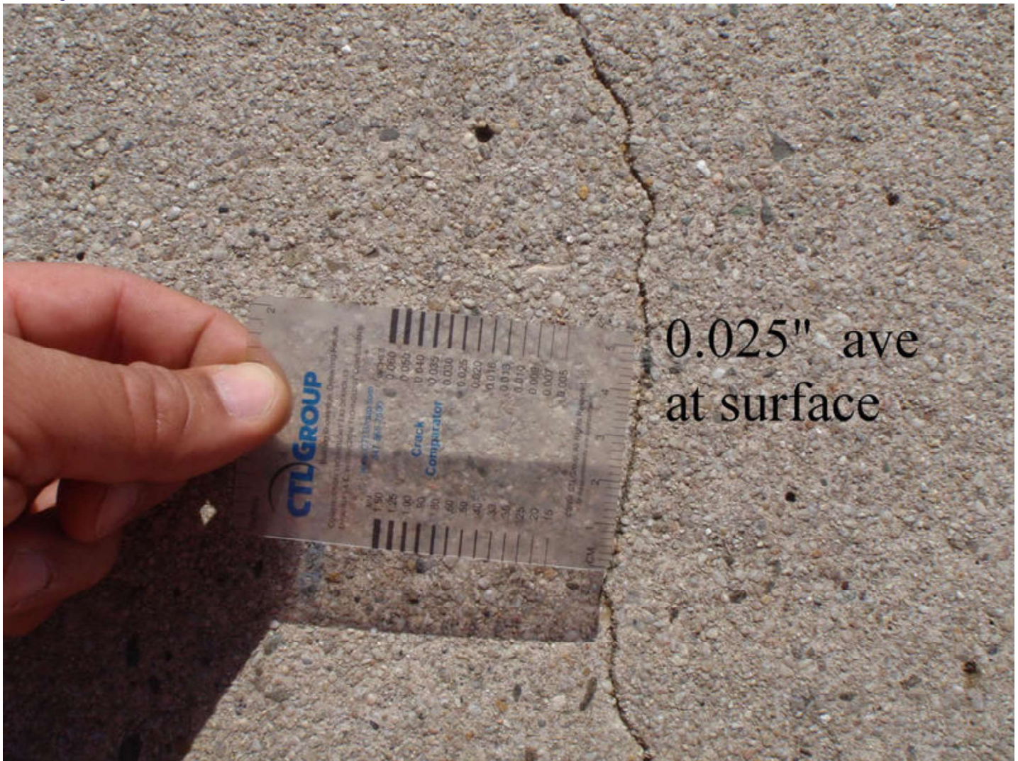
Photo #2 Typical deck crack size.
