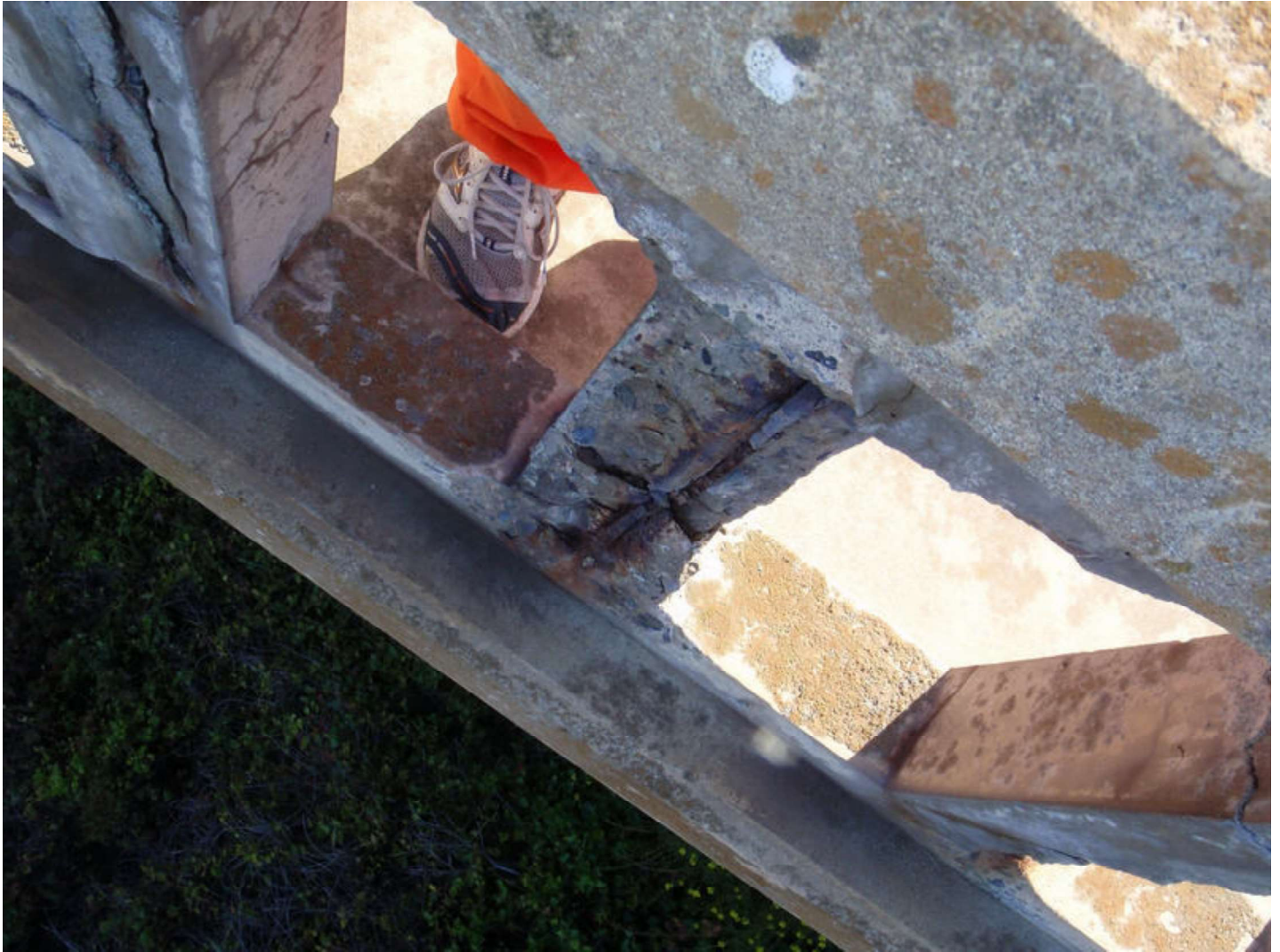
Photo #6 Gross deterioration of bridge railing.
