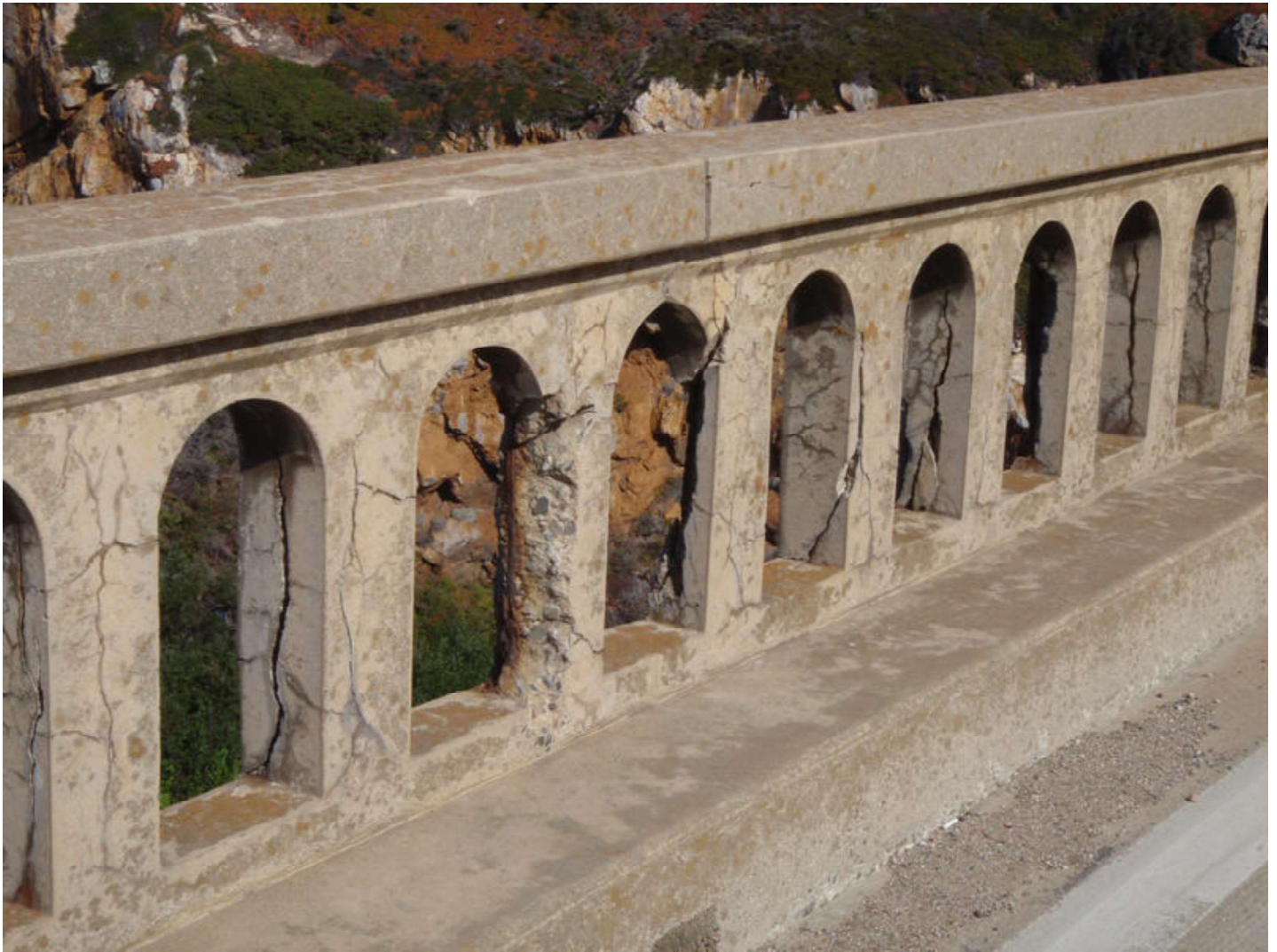
Photo #5 Gross deterioration of bridge railing.
