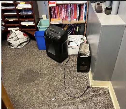
Worn out carpeting
