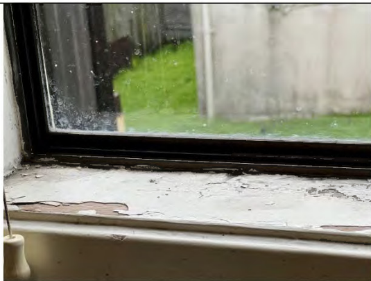
Window sill paint peeling
