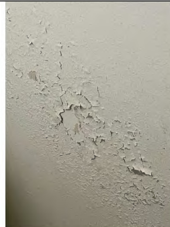
Kitchen paint flaking/peeling
