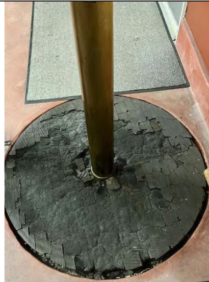
Poor condition of fire pole landing pad
