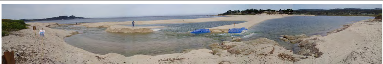
Temporary sandbags and tarps were used to raise the lagoon water level in Summer 2006
