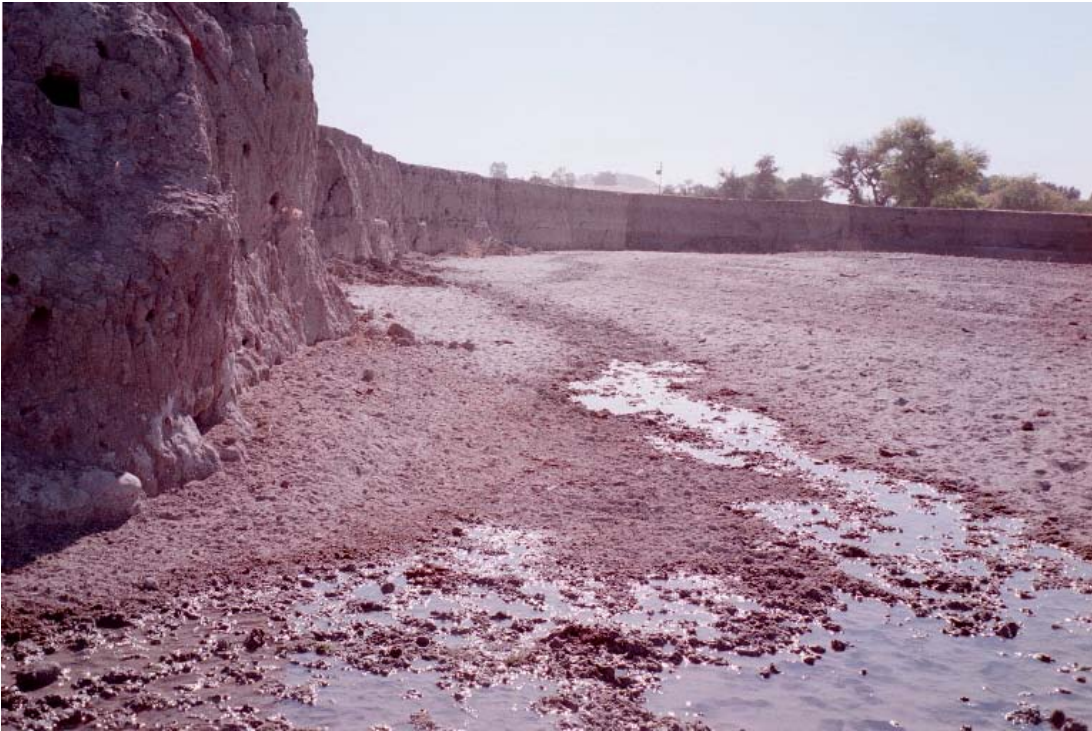
Photo 4.2 Cholame Creek erosion in a braided channel. Location is downstream of confluence with Little Cholame Creek. Riparian vegetation has disappeared.
