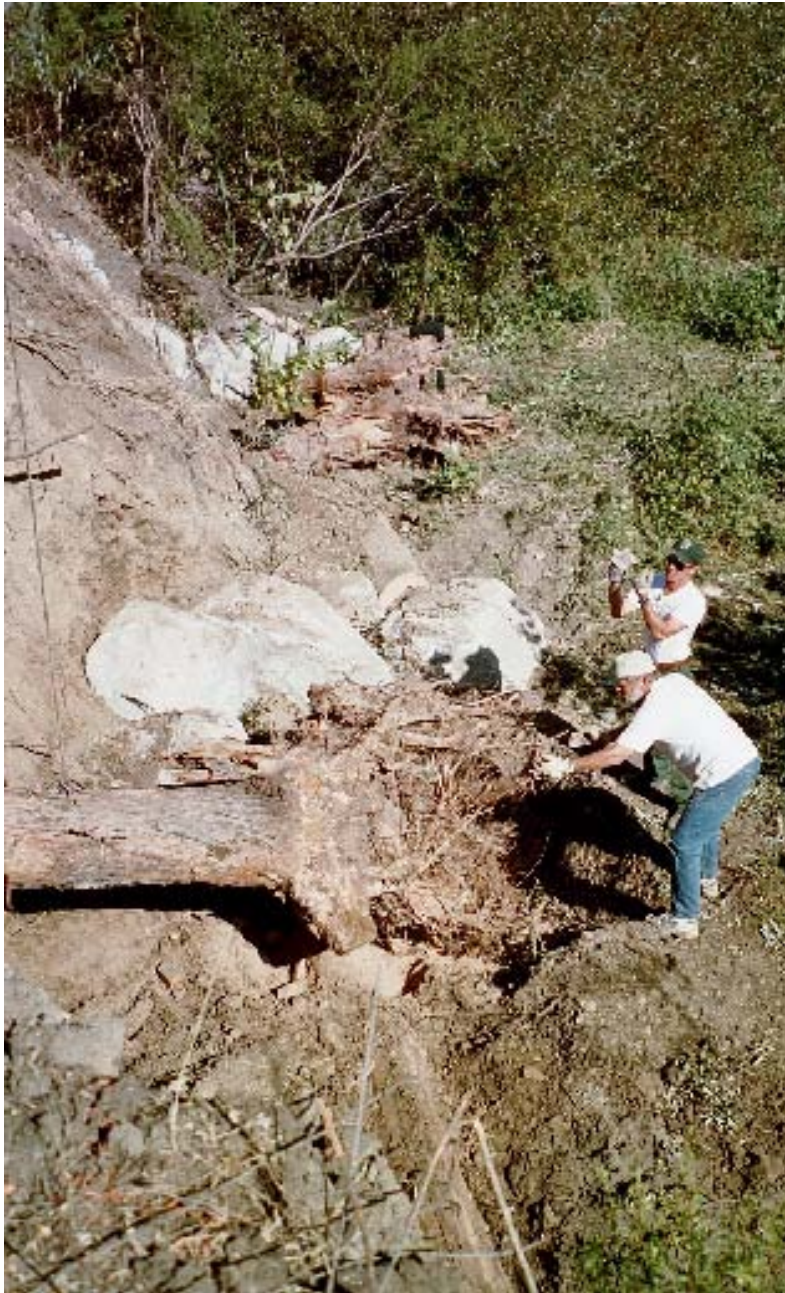
Photo 7.8 Department of Fish and Game staff assists landowner in maneuvering rootwad at US-LT RCD designed channel restoration
