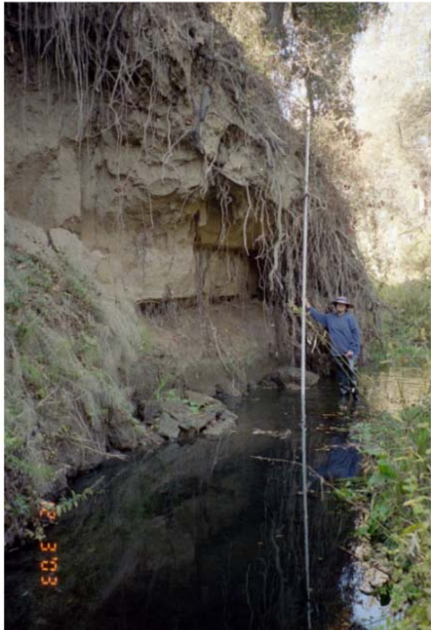
Photo 4.18 December 2003 survey shows 4 feet of bank erosion
