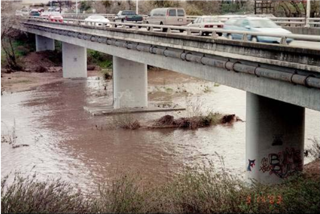
Photo 4.21 Salinas River, 13 th Street Bridge, after rainstorm, winter 2003
