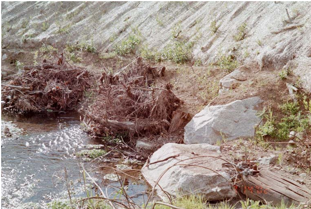
Photo 7.10 Creek Bank Stabilization and Restoration using rootwads, boulders and logs designed by RCD.
