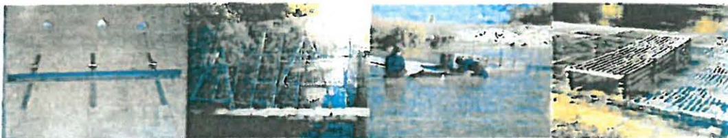
Figure A-1. Photos of a section of substrate rail prior to installation (left), rigid weir installed in the Stanislaus River (left-center), technicians installing a resistance weir panel (right center), and modified fish passage resistance panel.
