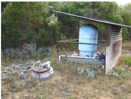
Groundwater well used for residence and for cattle watering in southern portion of site
