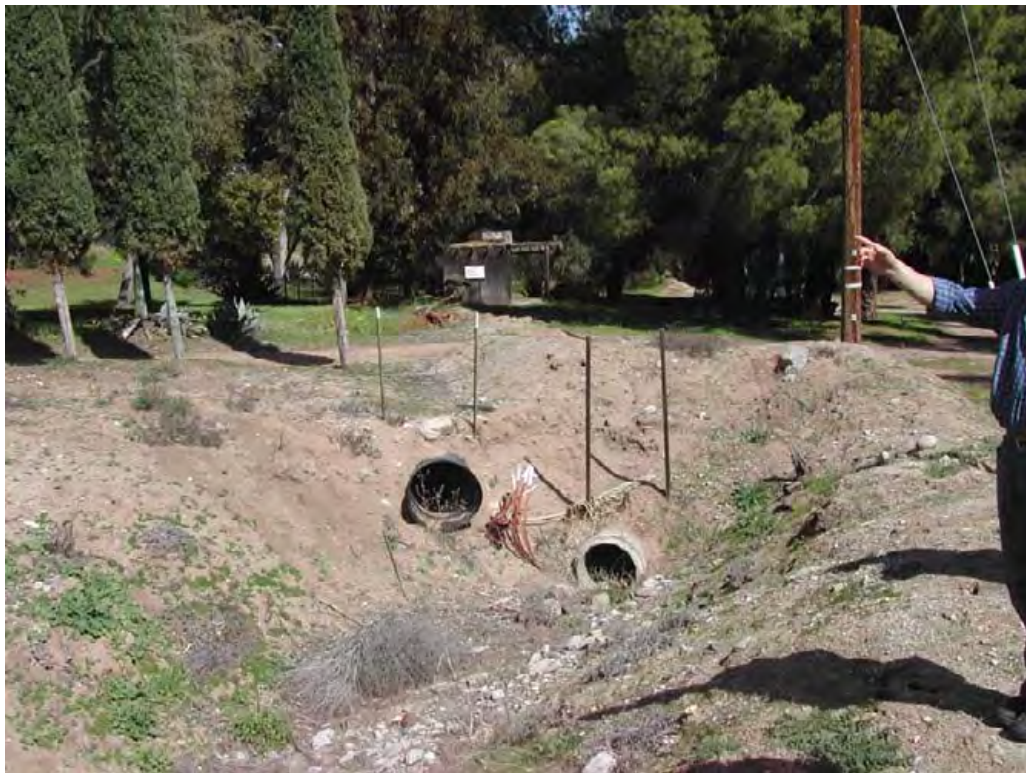
Photo 8: Main drainage channel looking downstream; culverts located upstream of the existing hot springs pools
