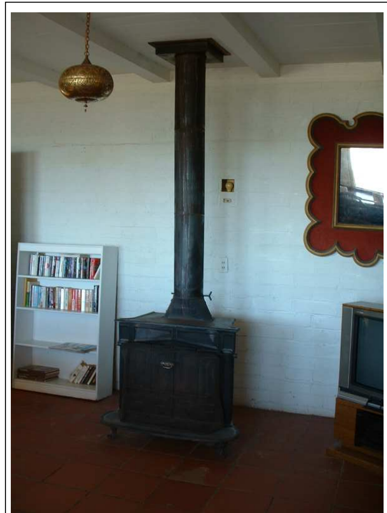
Photo 29: Interior view of the wood stove in snack bar.
