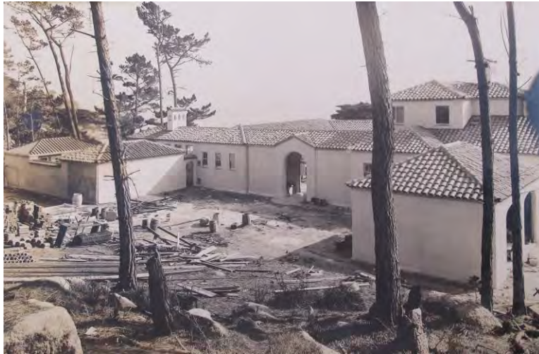
The Charles W. Clark house under construction, circa 1919. Today known as the Tobin-Clark house, it was designed by Bakewell & Brown. (Monterey County Planning Department collections)
