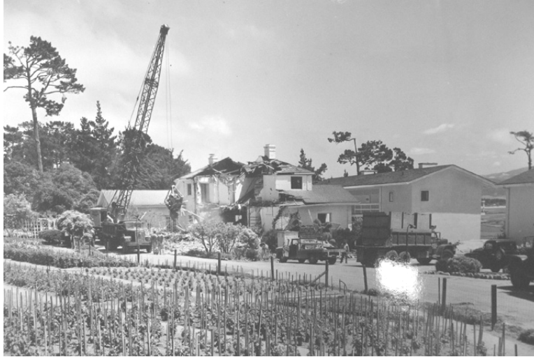
Demolition of Samuel F. B. Morse house near the 18th hole, 1965. The Portola lodging facility is at right of the house. (Courtesy the Pebble Beach Company Lagorio Archives)
