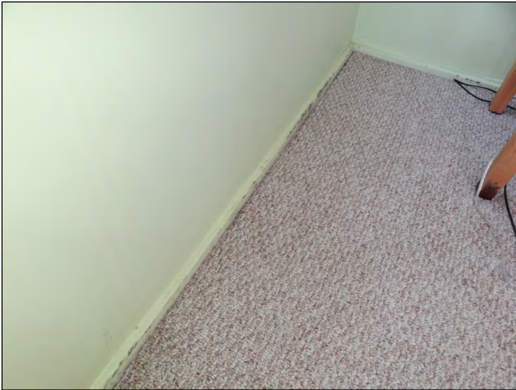
Mold growth on baseboard in master bedroom
