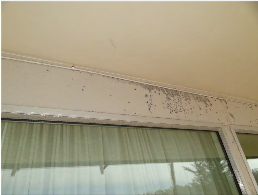
Suspect mold growth on outside of bedroom wall
