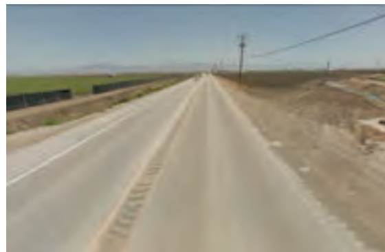
The shoulders of Blanco Road are commonly covered in dirt.
