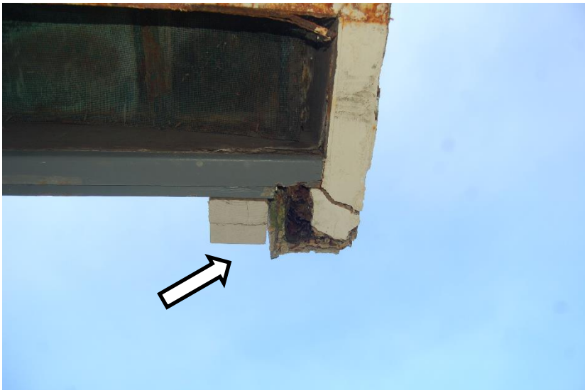
Photo 12 Framing deterioration at northwest corner of deck.
