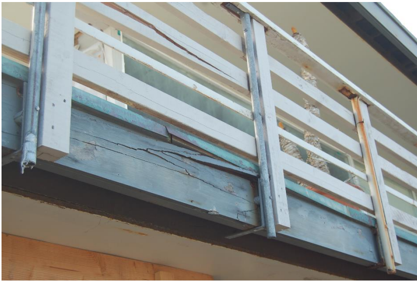
Photo 13 Deterioration and splitting at deck edge.
