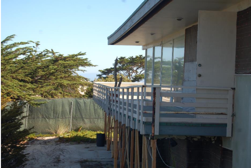
Photo 9 Sagging deck and handrail along upper level west face.
