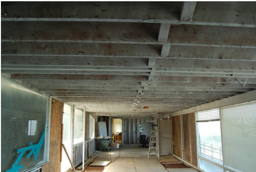
Photo 16 Finishes removed around the upper level bath, but still in place in the addition, visible to the rear left.
