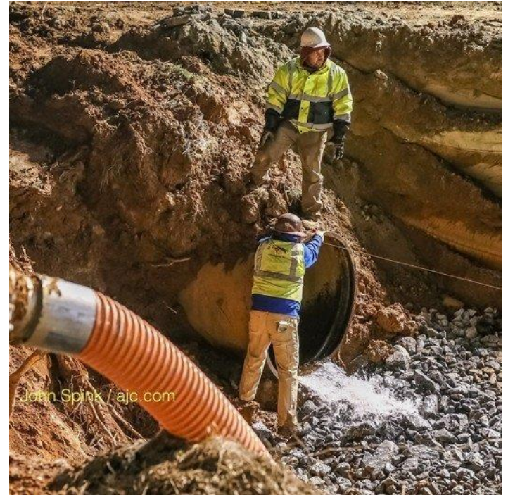
2018 Atlanta Water Main Break
